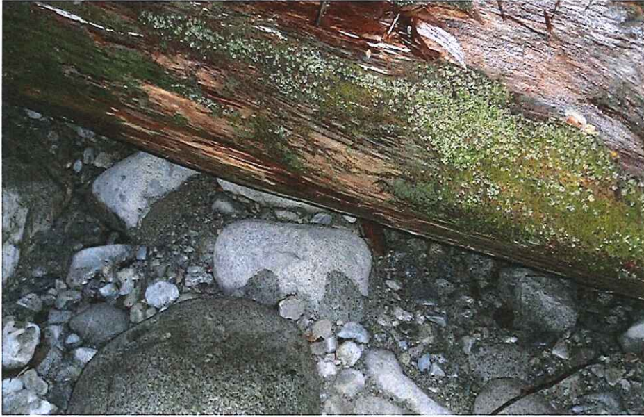
CK2176 Undermining scour left ban...
